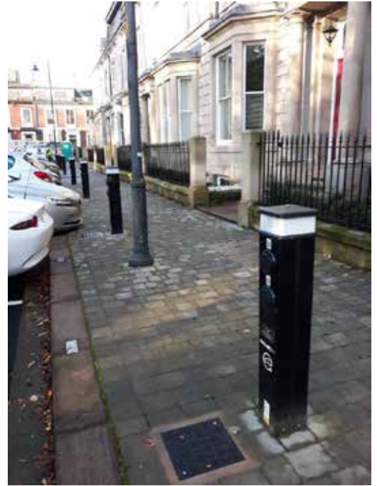
Charge point bollards at Portland Place, Carlisle
