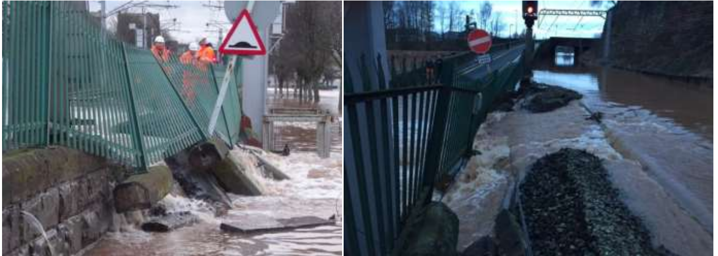
Photographs 9 & 10: Wall along railway at entrance to Viaduct Estate that collapsed during the flood event
