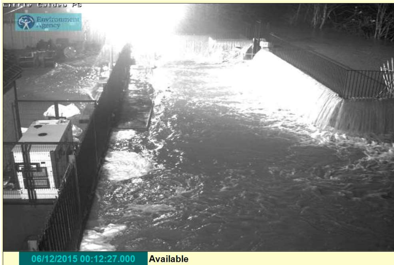
Photo 7: Little Caldew Pumping Station.
