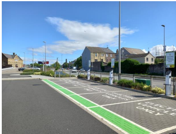
Image 6: An image of the electric vehicle charge points at Workington Train Station
