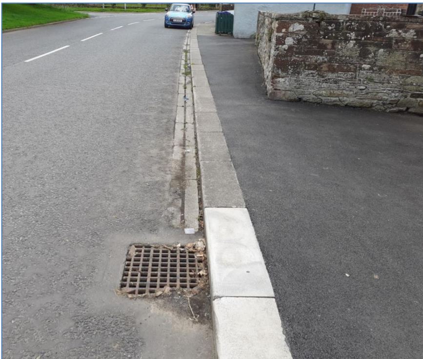
Figure 11. Channel drainage outside Rose Cottage and Joiners Shop, water in this location was approx. 300mm deep.
