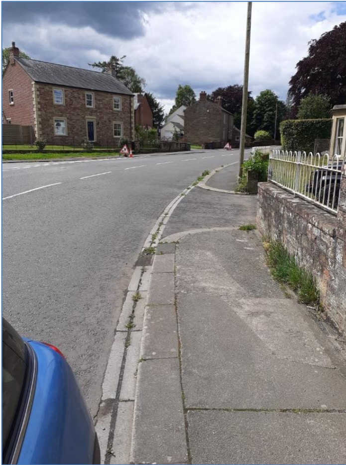
Figure 10. Highway channel drainage outside Cottage Meads and Carel Cottage
