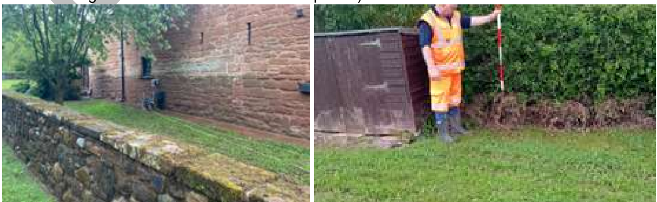
Figure 13: Wrack/water marks on property (left), EA checking flood extent levels (right)
