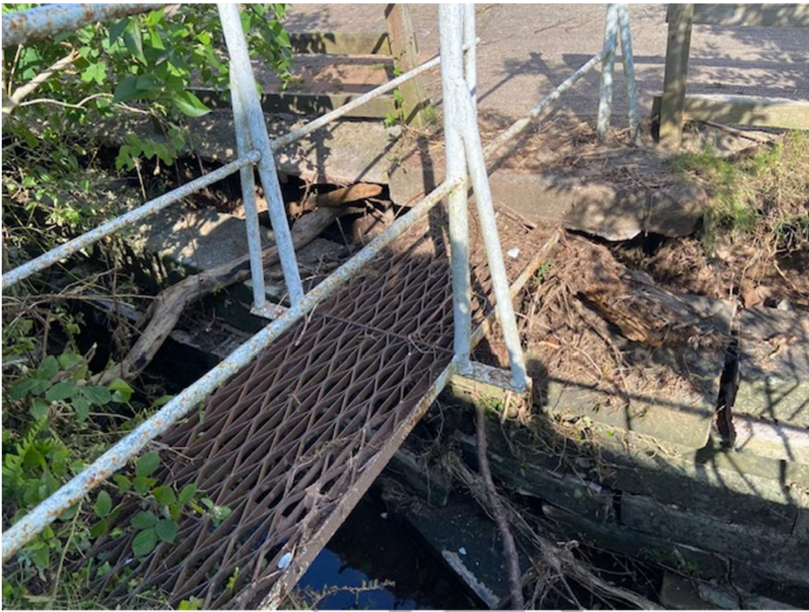
Figure 31: Footbridge accumulating debris
