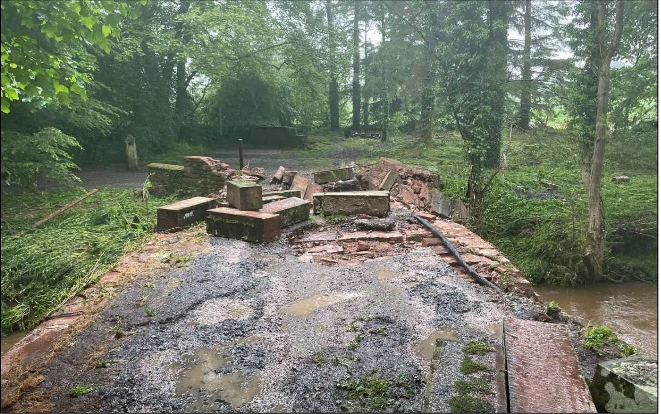
Figure 21: Partially collapsed access bridge at Roewath. Photo taken on 24/05/2024.
