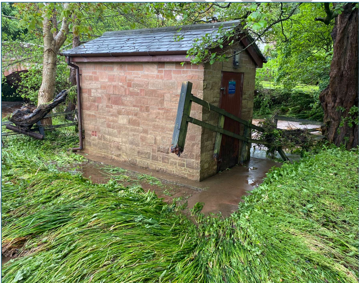
Figure 27: The kiosk of the Environment Agency river gauge. High water mark is faintly visible on the external walls, this was far clearer inside the building.
