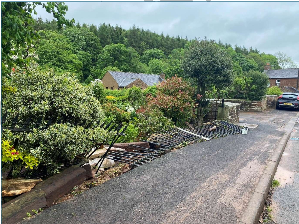
Figure 25: Boundary wall and fence at Stockdalewath pushed over by flood water
