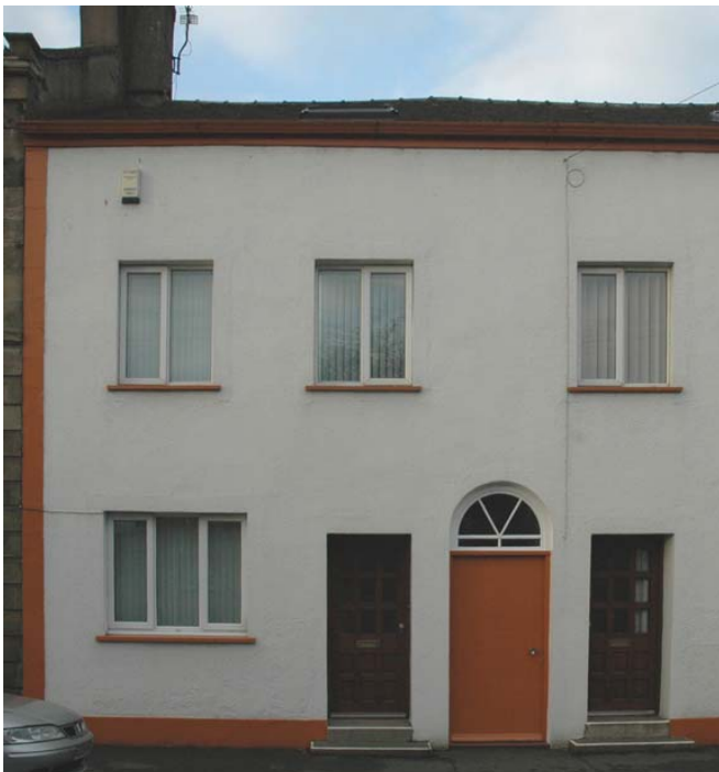
Loss of original features (non smooth wall finish, windows and doors) resulting in loss of architectural and historic interest
