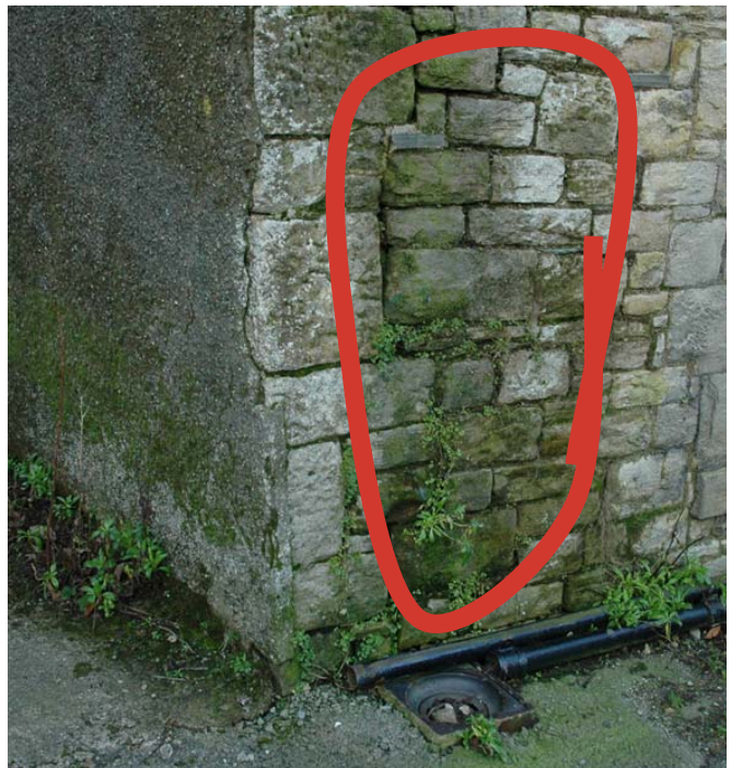
Saturated & damaged stonework due to missing downpipe
