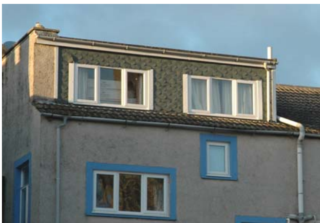
Inappropriate full-width dormer
