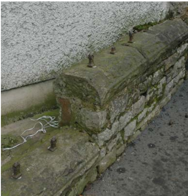
Evidence of lost original railings
